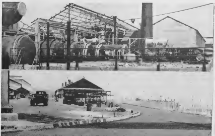
The old No. 3 evaporator plant is uprooted to make (Bottom picture) both the old road, left, and the new room for new storehouse space (top picture). This road, right, area shows. New section of shop will straddle space (16) will be warehouse space plus 500 sq. ft. of old road, while new road swings down past No. 1 & No. 2 Finger Piers.
